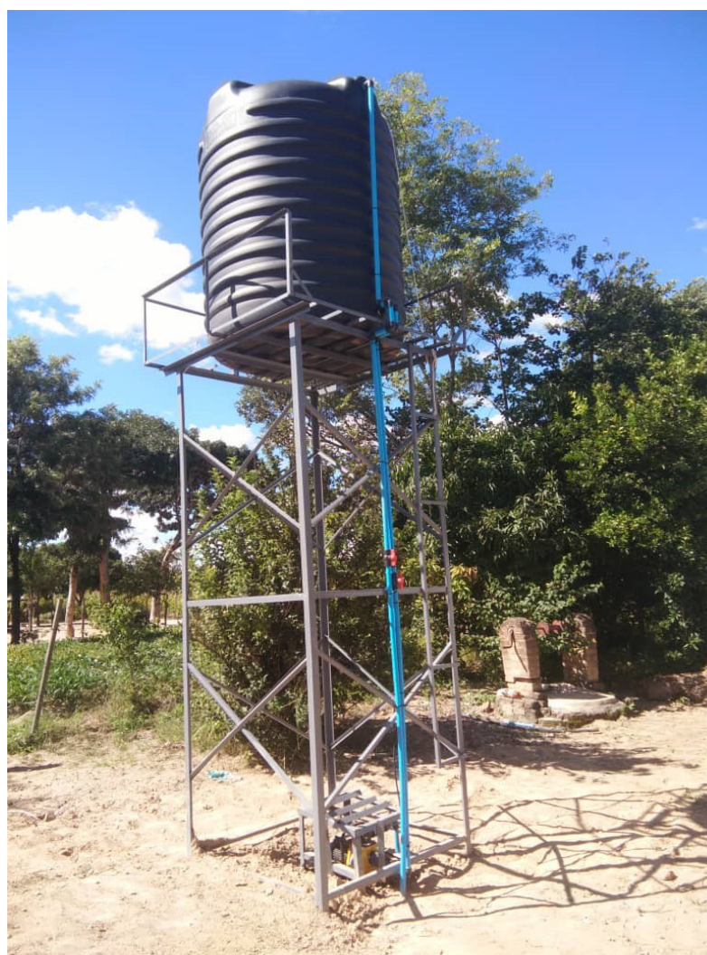
Installed water tank at the Mushroom Hub
